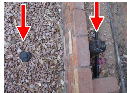
Main Plumbing Clean Outs
