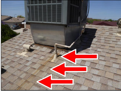
Unit 2 - Condensation Leak
