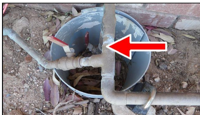
Main Water Shut Off Valve
