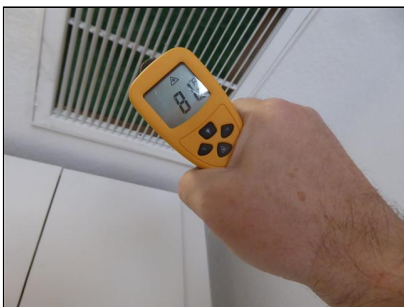
Unit 2 - Return Air Temp
