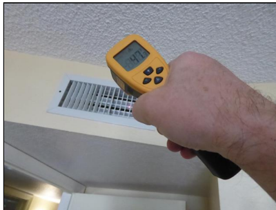
Unit 1 - Supply Air Temp
