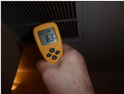
Unit 1 - Return Air Temp
