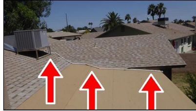
Unit 1 - Condensation Line
