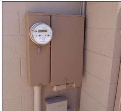
Main Electrical Panel
