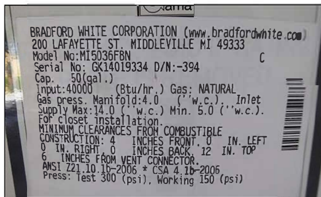
Water Heater ID Plate
