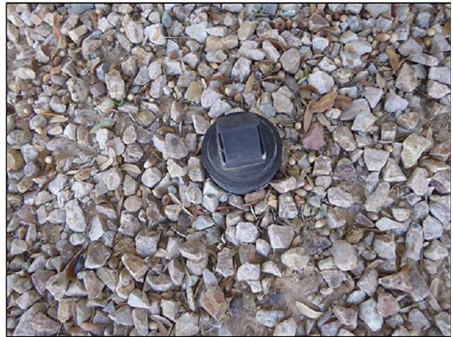
Plumbing Clean-out (front of home)
