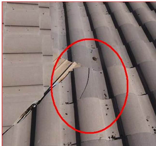
Cracked tile, 2nd level
