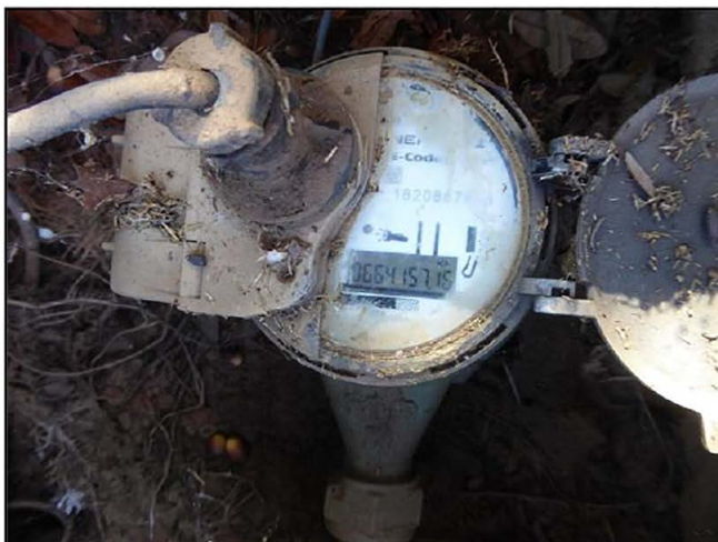
Main Water Meter
