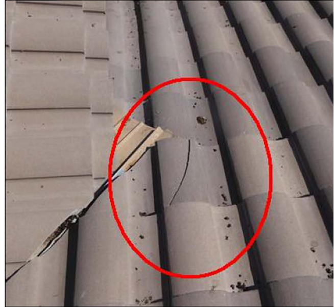
Cracked tile, 2nd level
