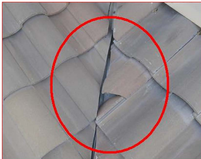
Cracked tile, front valley
