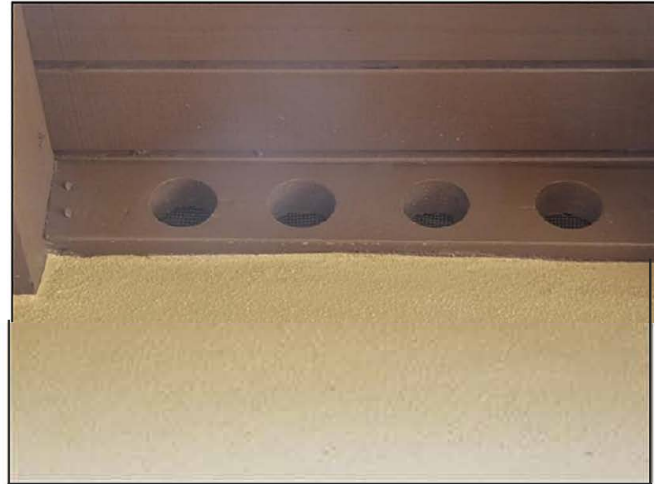
Attic - Soffit Vent
