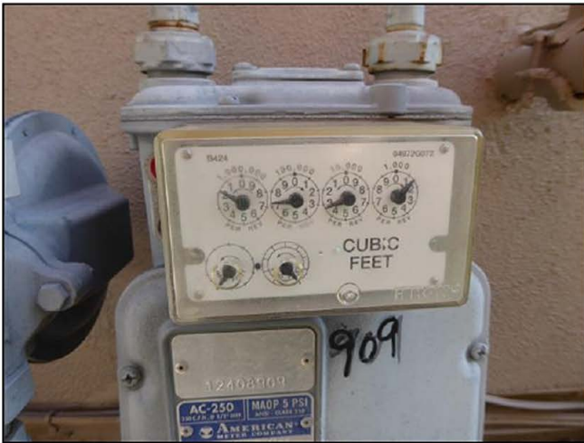
Gas Meter Reading
