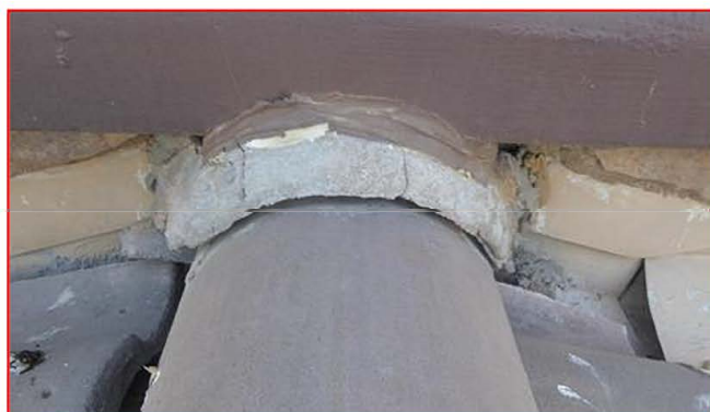
End cap cracking
