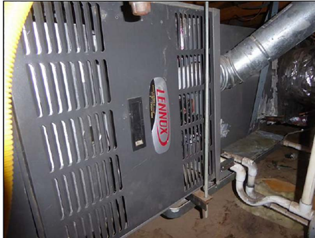
Gas Forced Air Furnace
