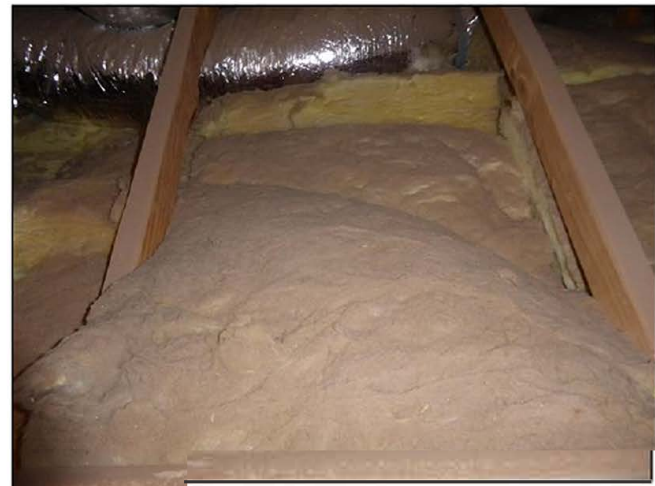
Attic - Batt Insulation
