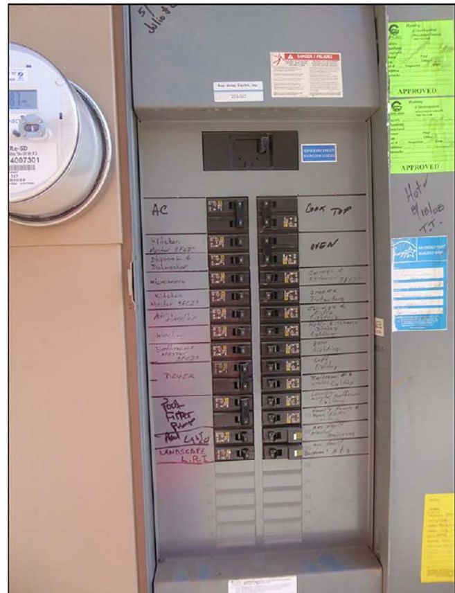
Main Electrical Panel
