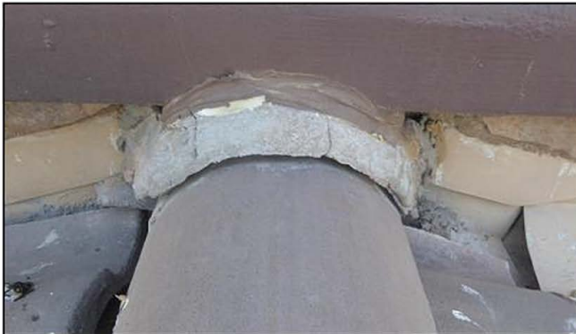
End cap cracking
