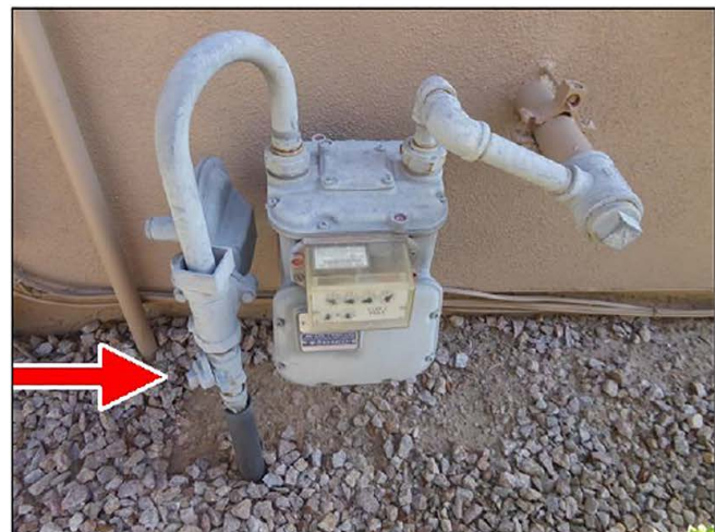
Gas Meter Shut-off Valve
