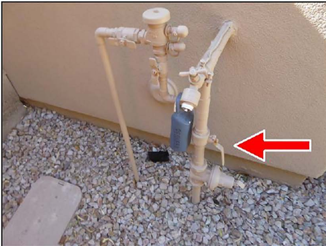
Main Water Shut-off Valve
